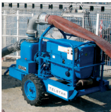
J4''D Station d'épuration.
